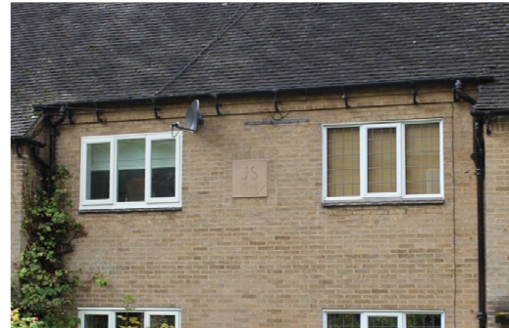
Right: Windows with a horizontal rather than vertical emphasis can be found on modern housing.
